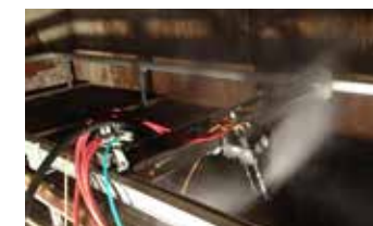
CONDENSER TUBE CLEANING
